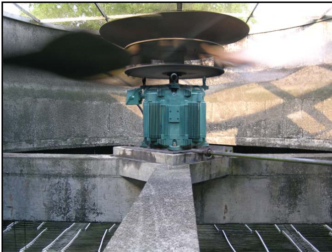
Fig. 10 PM Motor Installed in Place of Gearbox & Driveshaft
